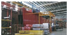
5-stage Jet Wash Powder Coating Lines
